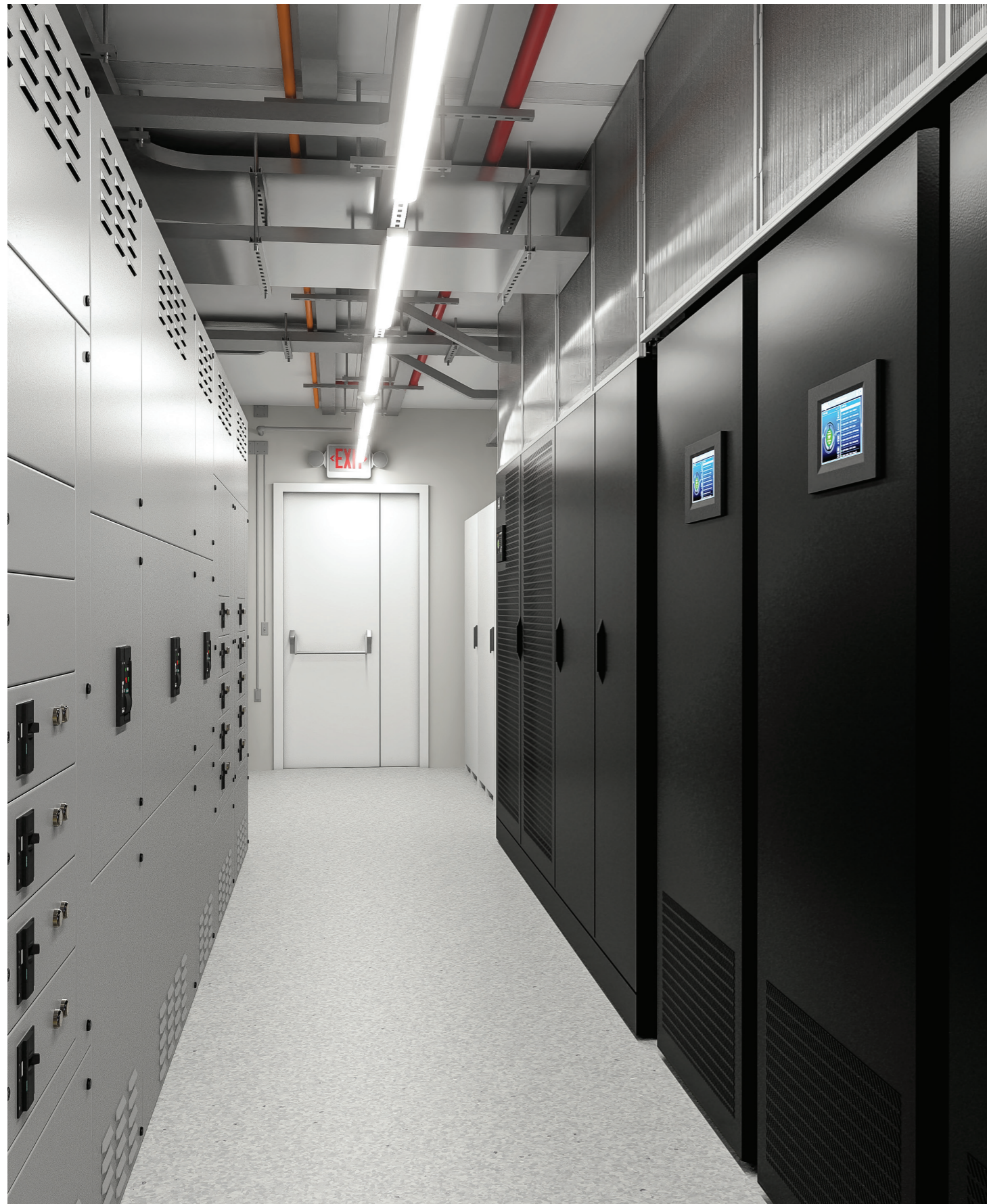
Vertiv Power Module 1000/1200 interior
