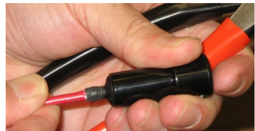
Figure 81. Checking Fuse holder/Load Lead Wire Connection
